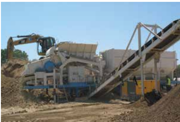
100 t/h mobile treatment plant (Photo: DigueELITE)
