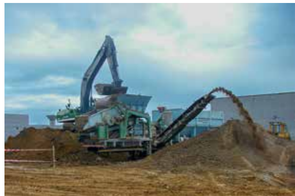
200 t/h mobile treatment plant (Photo: Lhoist)
