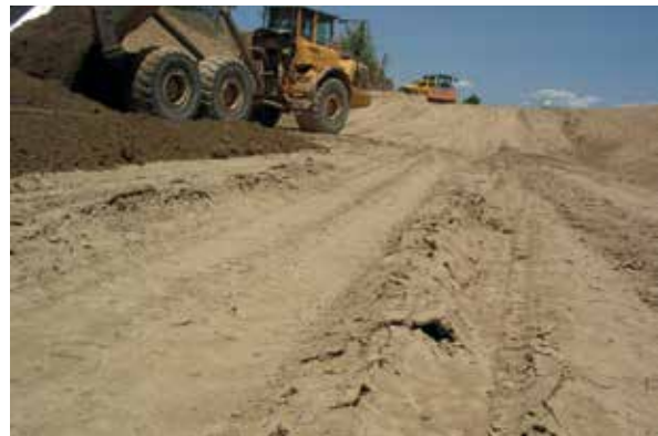
Example of creep caused during transport by a 6x8 dump truck on F1 soil at the Vidourle jobsite (Photo: DigueELITE)
