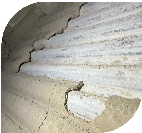
Example of fouling in an industrial boiler system
